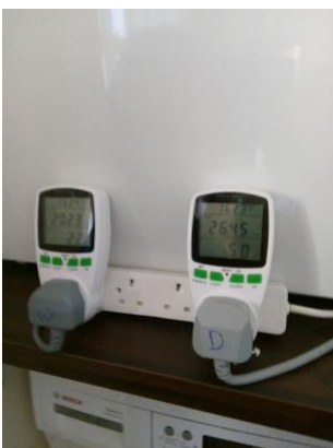
Picture 5: Electricity meters installed on washing machine and dryer
