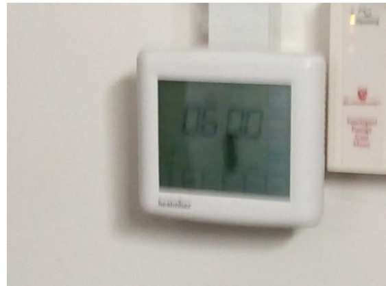
Picture 9: Controls for heat pump in a newly retrofitted house
