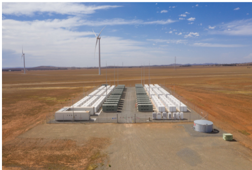
Hornsdale Power Reserve 129 MWh, 100 MW, 56 M€
