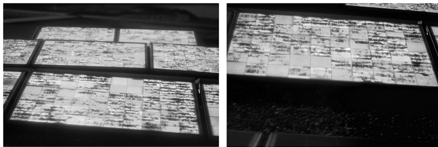
Fig. 10. a, b: TW-EL image of hail affected modules of plant 1 (glass not broken, ~ –30% power loss due to micro cracks).
