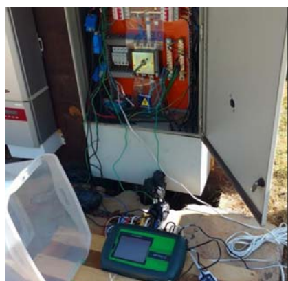
Fig. 4 Energy meter connected to the output of a three-phase solar inverter in Tanquinho solar power plant, Brazil
