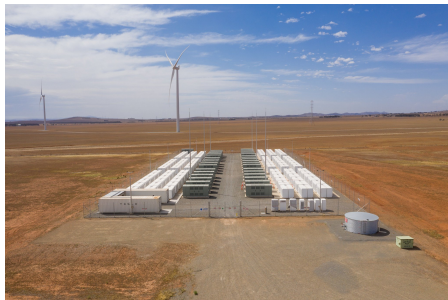
Hornsdale Power Reserve 129 MWh, 100 MW, 56 M€
