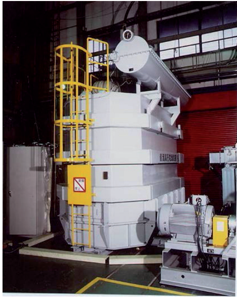
Fig. 6.22. High voltage power supply with oil insulation
