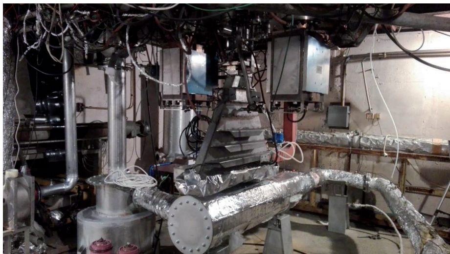
Fig. 5.7. View of the flue gas treatment installation based on the hybrid electron beam method
