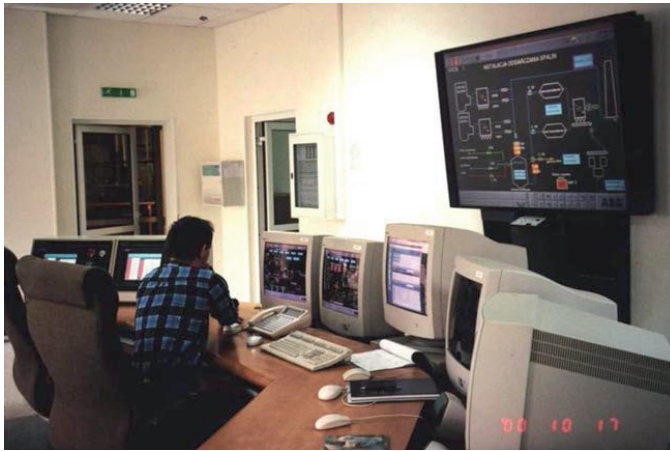
Fig. 6.29. Control room of flue gas treatment facility located at Pomorzany Power Station
