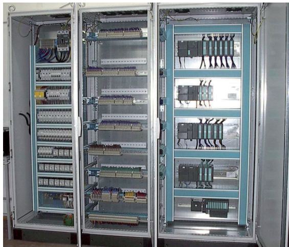
Fig. 3.19. Control panel with fuse and breaker unit, connection unit, and microprocessor and interface module units
