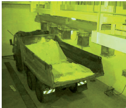
Fig. 6.35. Part of the flue gas treatment facility responsible for by-product collection and transportation
