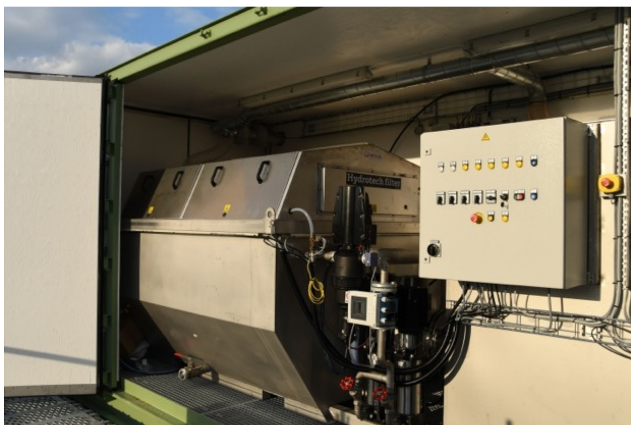
Figure 8: Hydrotech filter unit used for carbon Extraction at Westewitz Case Study 1
