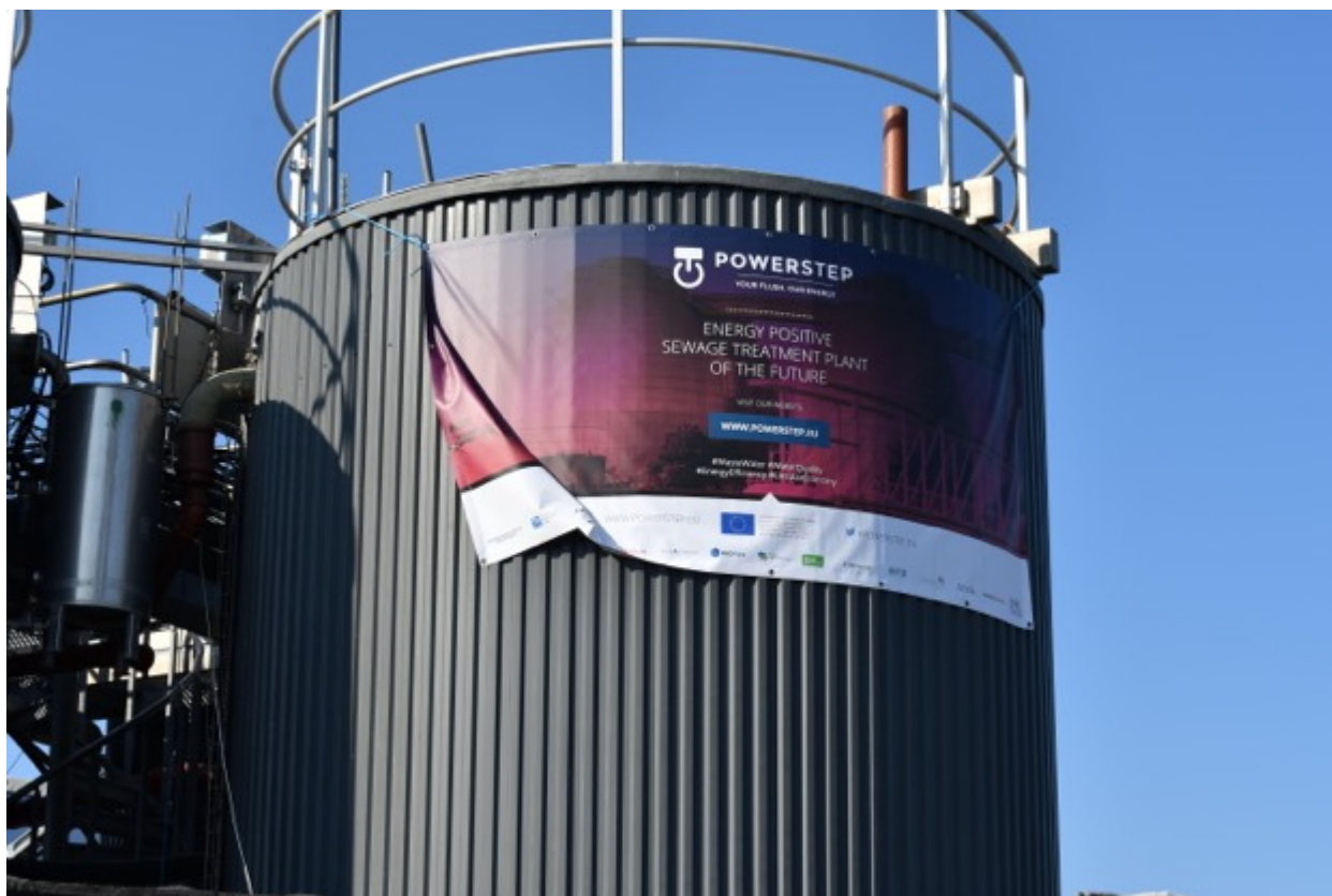
Figure 11: MBBR reactor for main stream Annamox at Sjölanda Case Study 2 site
