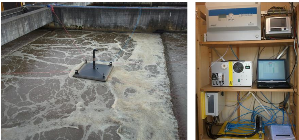
Figure 21: Floating gas hood on a reactor (right) and monitoring unit (left)
