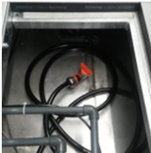
Figure 7: Drain Pipeline under floor panel in the left corner of the Service Section (as seen from the Cold Porch) under the table
