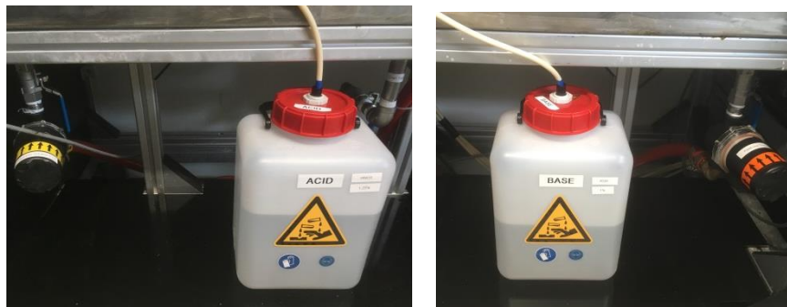
Figure 7: Acid and Base Tanks within the NDS
