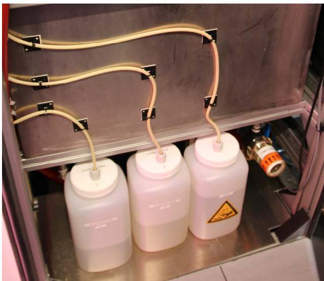
Figure 4: NDS Rack – Stock, Acid and Base Solution Tank 2
