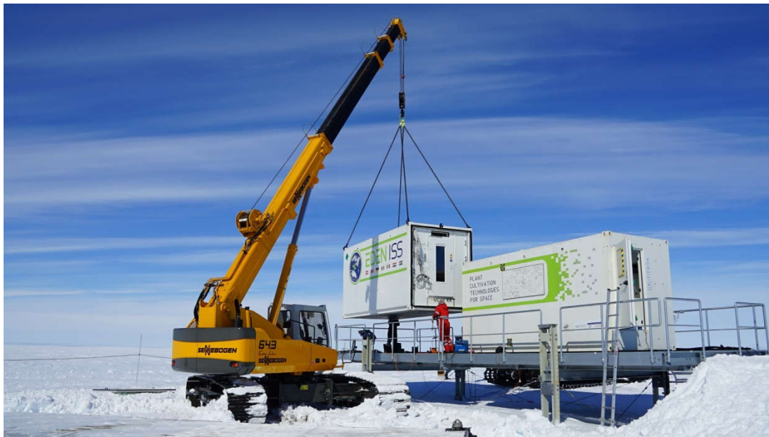
Figure 3: Installation of the EDEN ISS containers onto the previously installed elevated platform.
