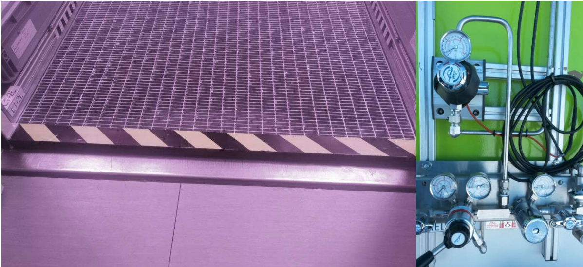
Figure 12: (Left) Floor installed door bar with insulating rubber. (Right) CO 2 distribution system with installed secondary regulator heater.
