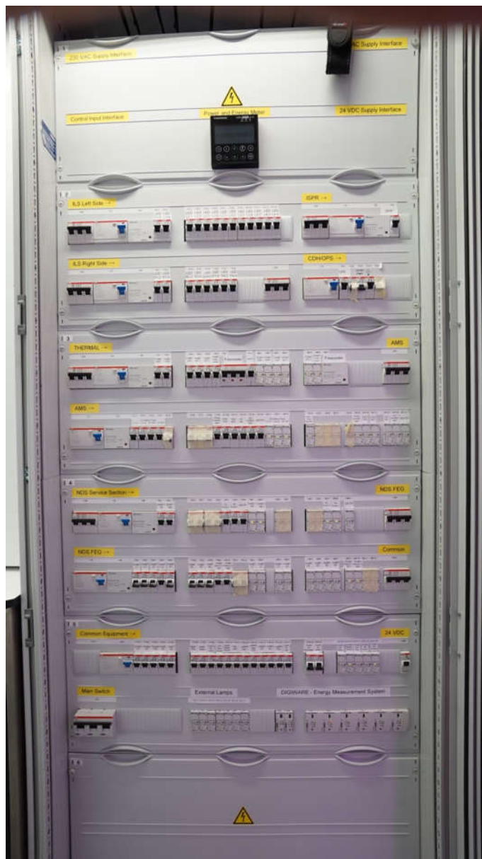
Figure 1-2: Main power box, as built.
