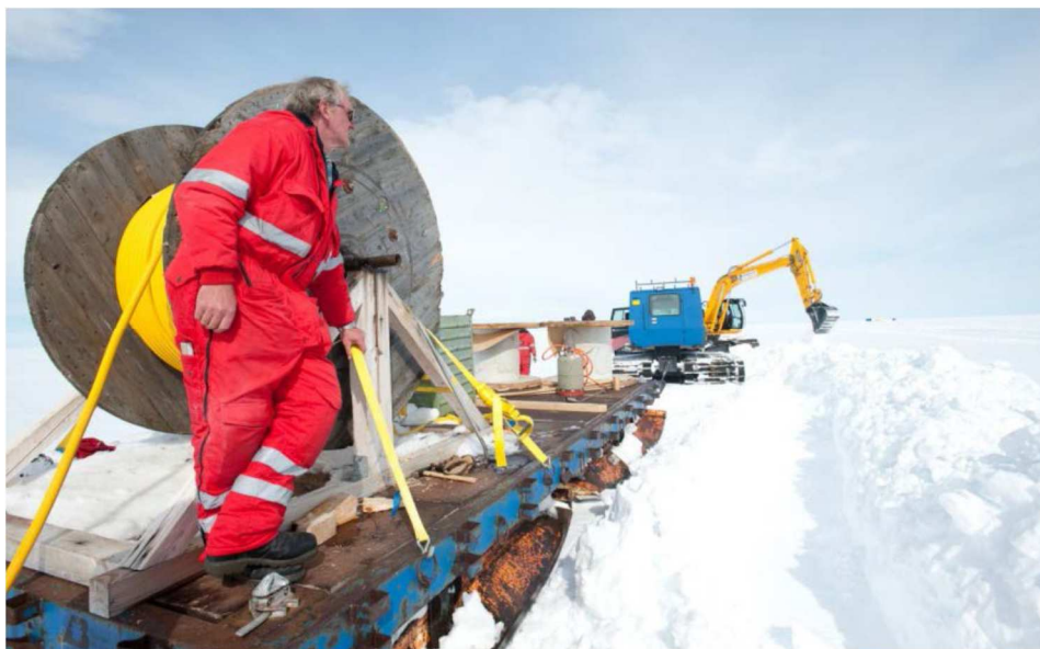
Figure 15: Heavy gauge electrical cable being laid for the NM-III Air Chemistry Laboratory. A similar cable and procedure is baselined for the MTF.
