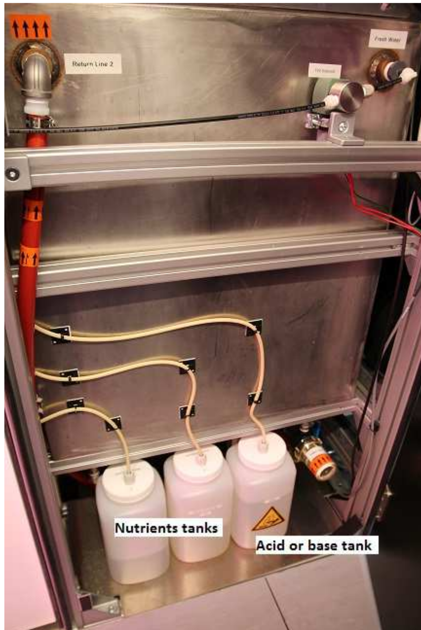
Fig. 149 NDS Rack – Tanks
