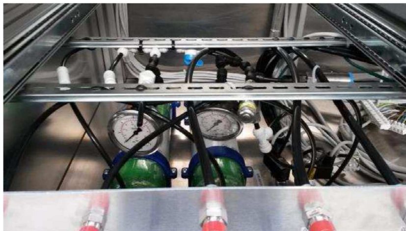
Figure 153: CO2 bottles inside the lower left side of the Main Utility Module
