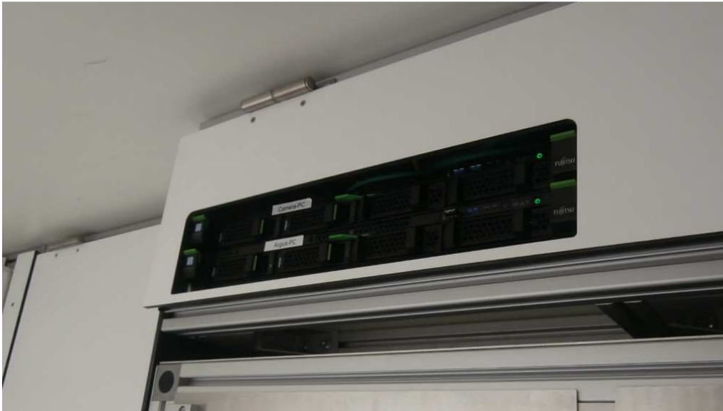
Fig.33: CDHS Computers installed above the ISPR Rack
