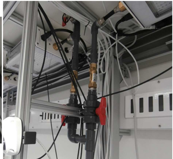
Figure 26: Led Panel Water Cooling Line
