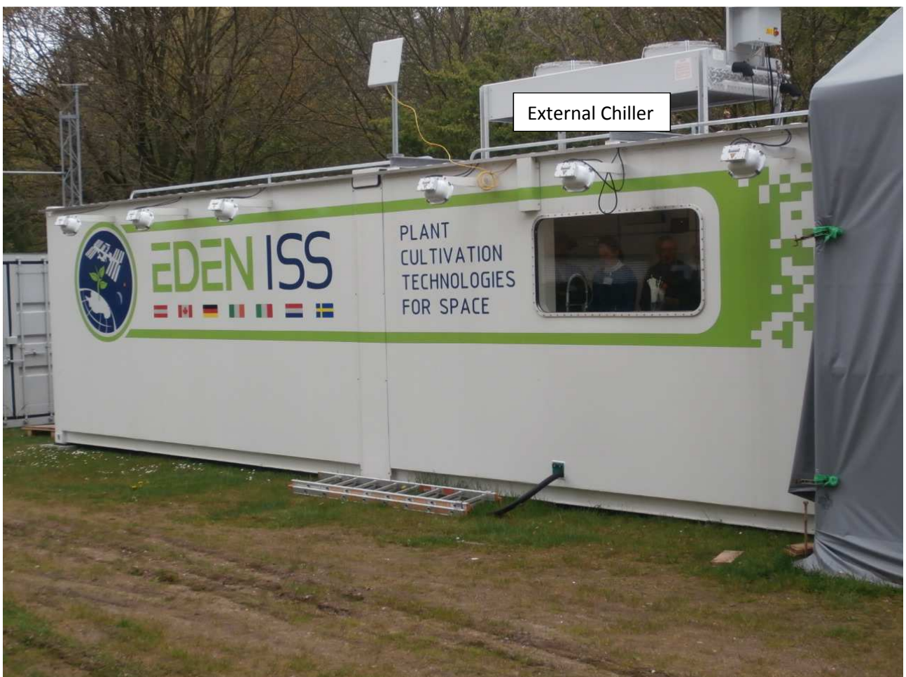
Figure 20: The External Chiller
