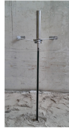
Figure 3-13: ASM as installed
