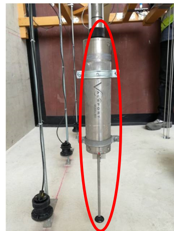
Figure 3-7: Electro-magnetic current meter as installed
