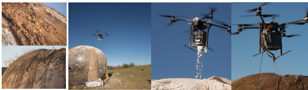
Figure. 2: From Left to Right Close ups on the matter surface adhesion and the drone spraying 2 kinds of clay mix over the formwork. January 2018. Test at the Barcelona drone center by the authors.
