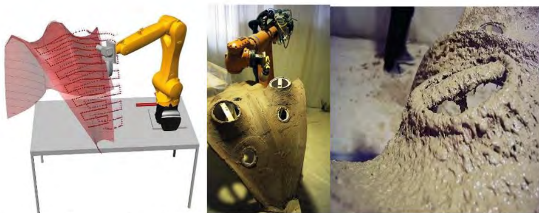
Figure 10. (a) Kuka PRC simulation of robotic trajectories after the first scan of the temporary formwork. (b) Middle layers of clay mix containing fibers applied by robotic spraying. (c) Close-up of the freshly projected fibrous clay mix robotically applied on the shell.
