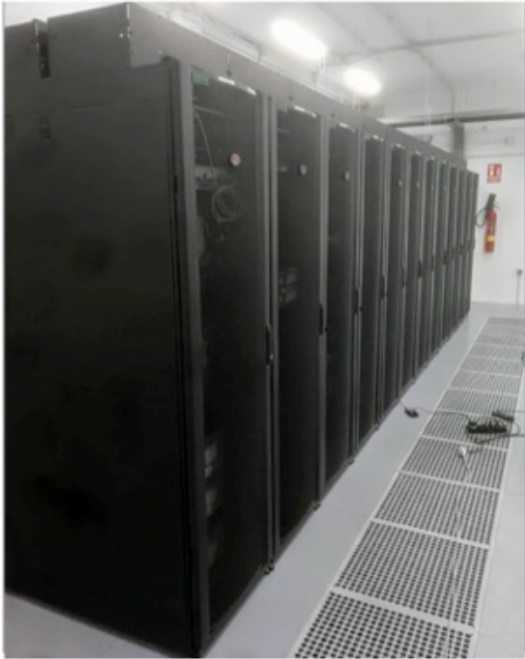
Figure 21: 5TONIC data centre
