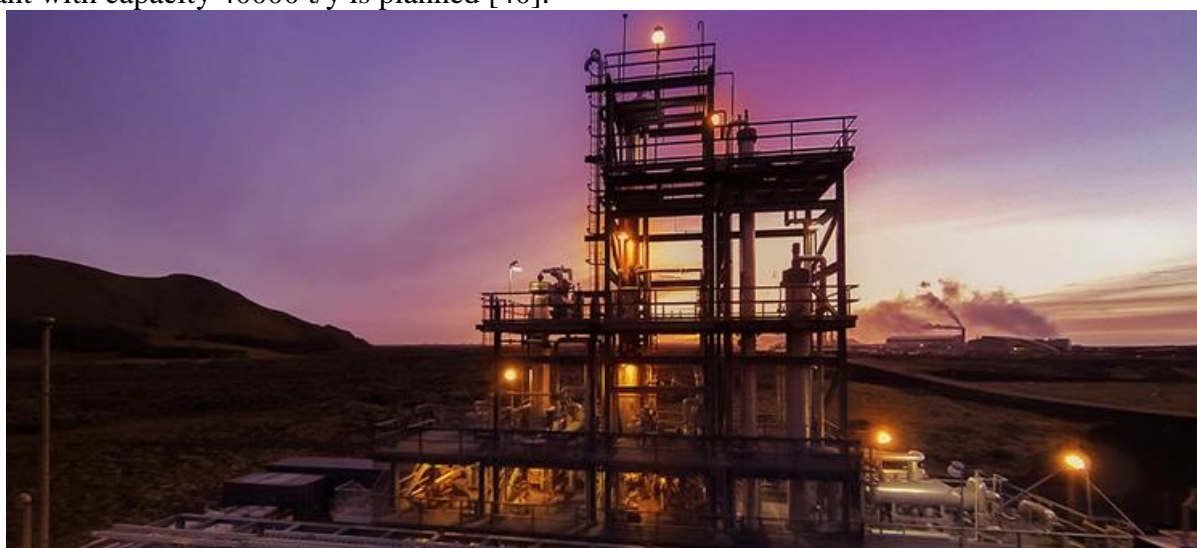
Figure 4-5: CRI's George Olah Renewable Methanol Plant in Svartsengi. World's Largest CO 2 Methanol Plant. Source: [41]
