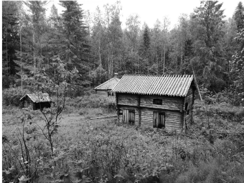
Fig.2 The historic wooden settlement of Jylhämä in the region of Vaala, Finland. This place it used to be a former outdoor museum along the Oulujoki River. After years, it was sold to privates that are today the owners. The buildings are in a serious state of abandonment. The vegetation has already started to surround the architecture. Timber structures are dramatically compromised. Now there are not any documentary actions of intervention for repairing this heritage, which is destined to disappear if specific restoration activities will not start soon
