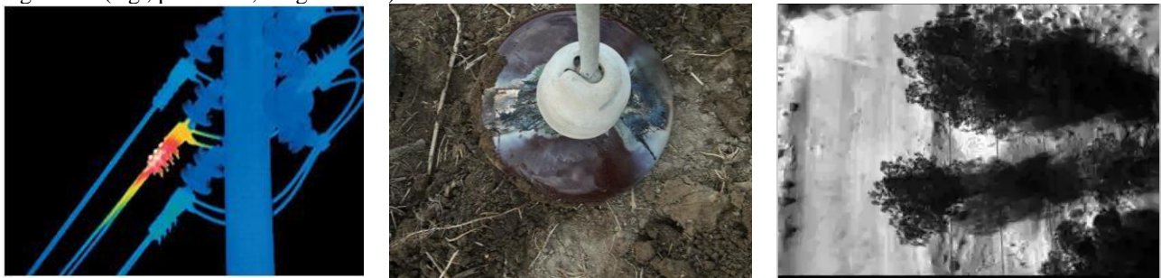
Fig. 4. Drone-based powerline inspection. (a) Detection of overheated insulator, (b) destroyed insulator, and (c) Powerlines as viewed by a thermal camera.
