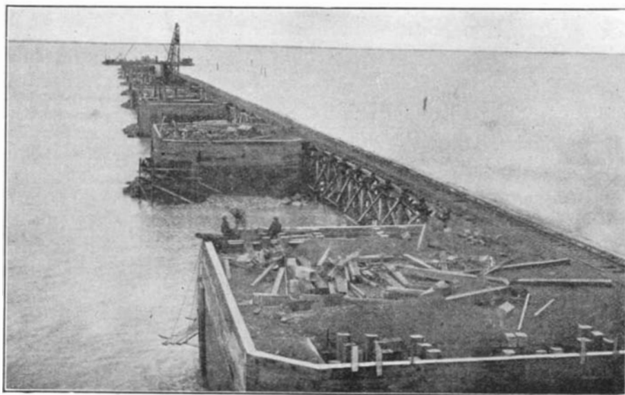
Looking toward new Hudson Bay ship channel, showing work in progress on bridge piers. In the foreground, hardwood and steel plate ice bulkheads are being placed
