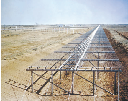
(a) Part of the master transmitter antenna at Lake Kickapoo, Texas, contributing to the AFSSS until 2013. (Public domain image, https://commons.wikimedia.org )
