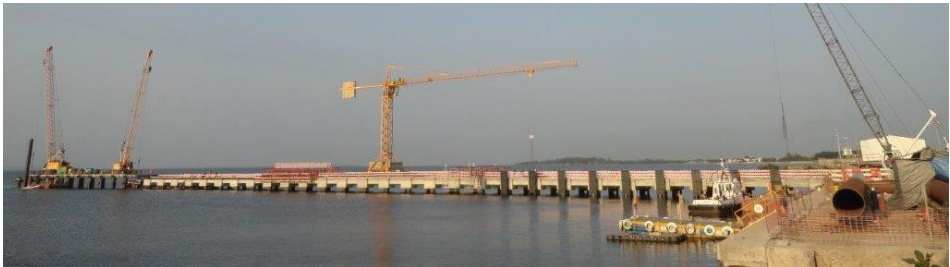
Figure 3: Jetty under construction. Stg.1 - Pile driving. Stg.2 - Temporary jetty movement. Stg.3 - Precast assembly. Stg.4 – Cantilever system. Stg.5 – Fenders assembly with a tower crane on tracks.
