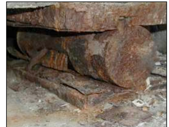
Deterioration of bearings
