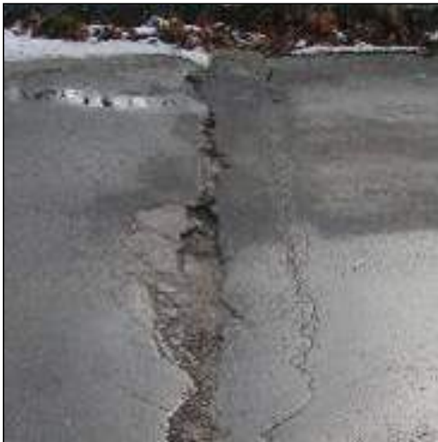
Differential settlements on the bridge-embankment transition
