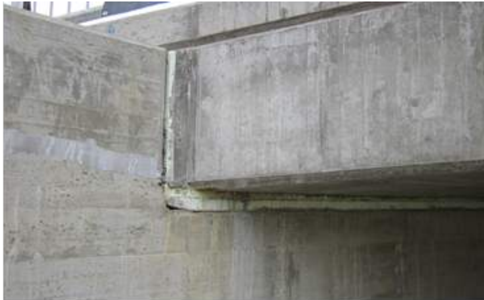
Gap between the top of the facing and bottom of the bridge superstructure (i.e. slab deck)
