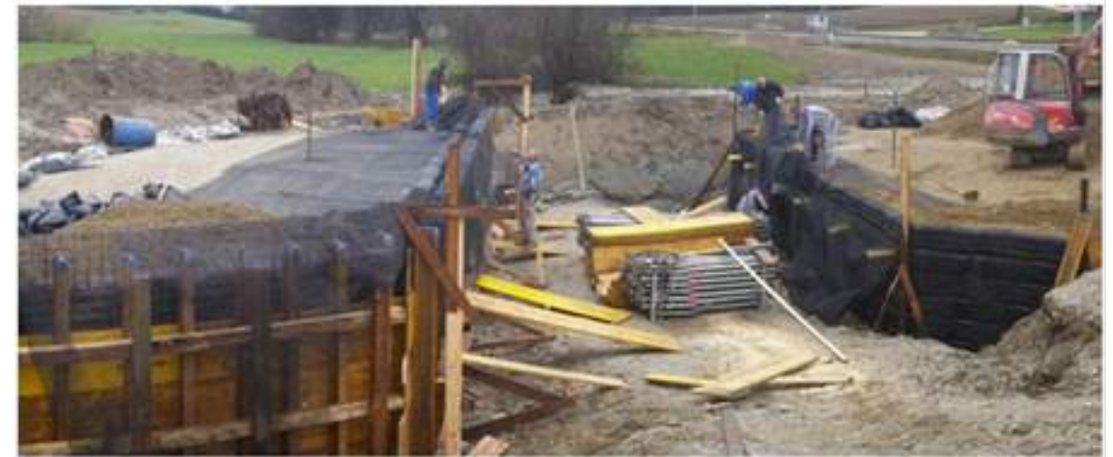
Construction of the GRS abutments by placing gravel bags on the shoulder of each layer and compaction of the backfill
