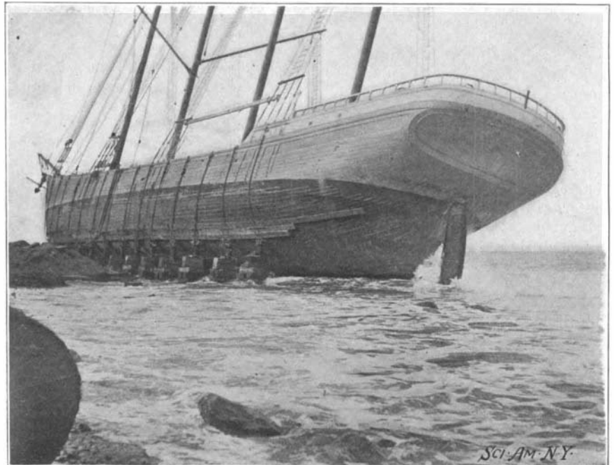
WRECKED SCHOONER "CAINE," SHOWING LINE OF HYDRAULIC JACKS BY WHICH SHE WAS LIFTED FOR INSERTING LAUNCHING WAYS.
