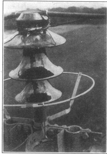
FIG. 14.—Insulator, protected by lower arcing ring, which flashed over successfully
