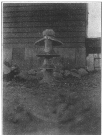
FIG. 15.—Insulator injured in head-piece by power arc. No upper arcing ring was installed
