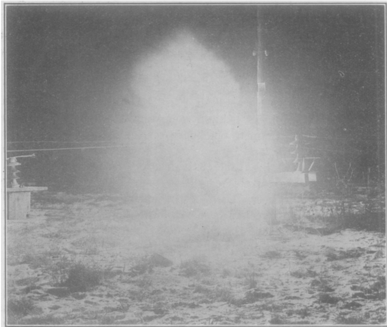
FIG. 8.—Night photograph of a 30,000-kw. 1200-ampere arc on an insulator equipped with arcing rings
