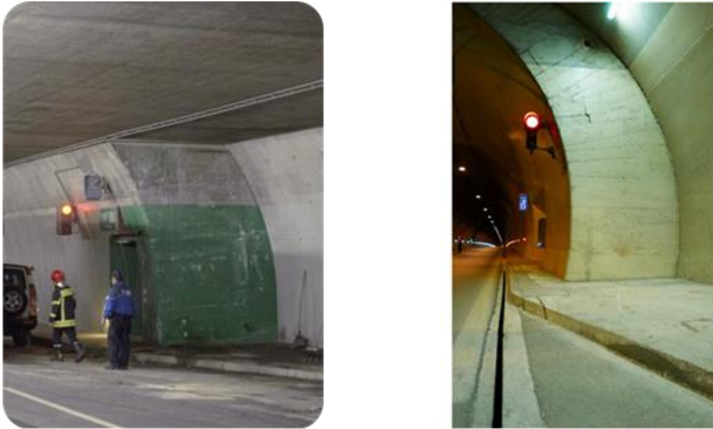
Fig 2 Left: the lay-by in Sierre Tunnel. (source – www.ecoroads.eu ). Right: similar situation (source: Hasani A., Albanian Roads Authority)
