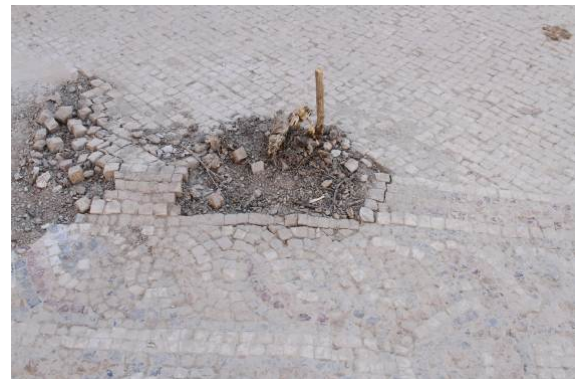
Figure 9 Bulge caused by plants
