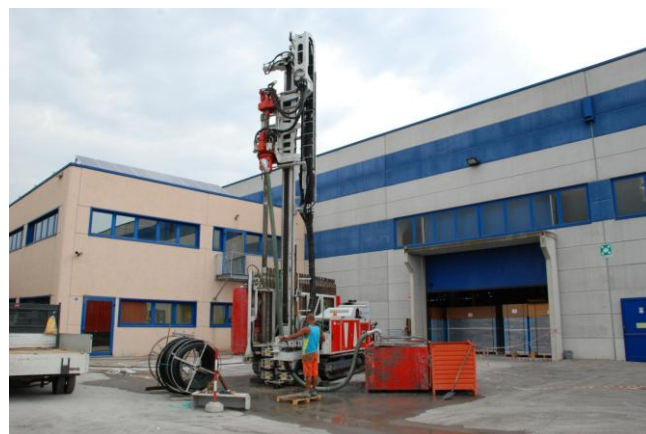
Figure 1: Drilling borehole heat exchangers by ENEREN at HIREF factory demo site, in Tribano, Padova
