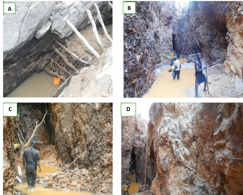
Figure 6. Deep and dangerous barite artisanal mining in Nasarawa state ((A)—potential pit wall failure supported by wooden props, (B–D) shows artisanal miners working at deeper levels). Photo credit: authors.
