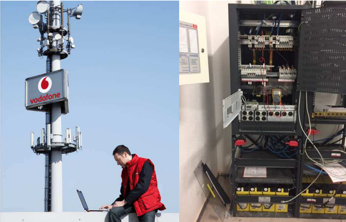
Figure 5. Outdoor and indoor equipment of a base station
