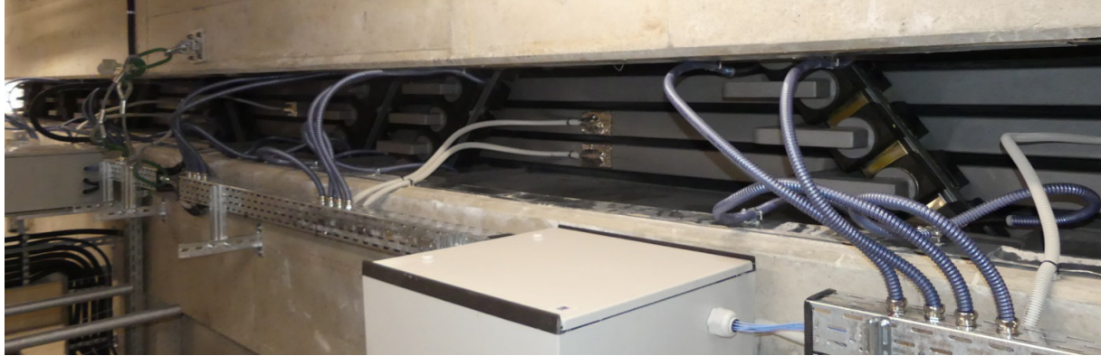
Fig. 7 Instrumented expansion joint
