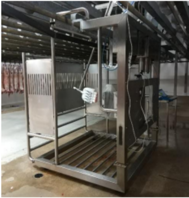
Figure 1 – Production Prototype installed in the chiller. The pusher arm is in the centre of the photo. The Marbl™ sensor is partially obscured.
