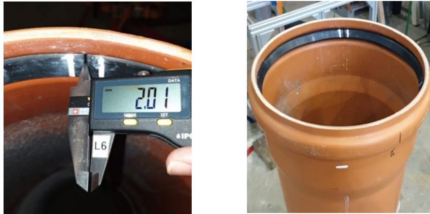
Figure 10. Left: crack measured with an electronic caliper. Right: location of damaged seal in PVC pipe at 6 o'clock
