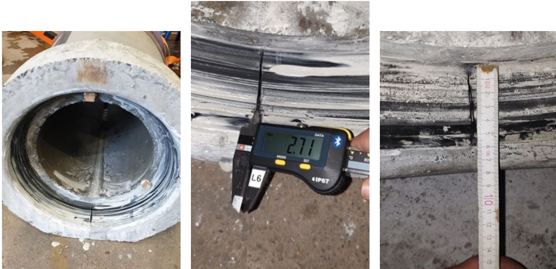
Figure 11. Left: defect in seal at 6 o'clock. Centre: measurement of the width of the crack (2.7 mm). Right: length of the defect in the seal 59mm
