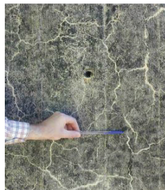
b) Map cracking [8]
