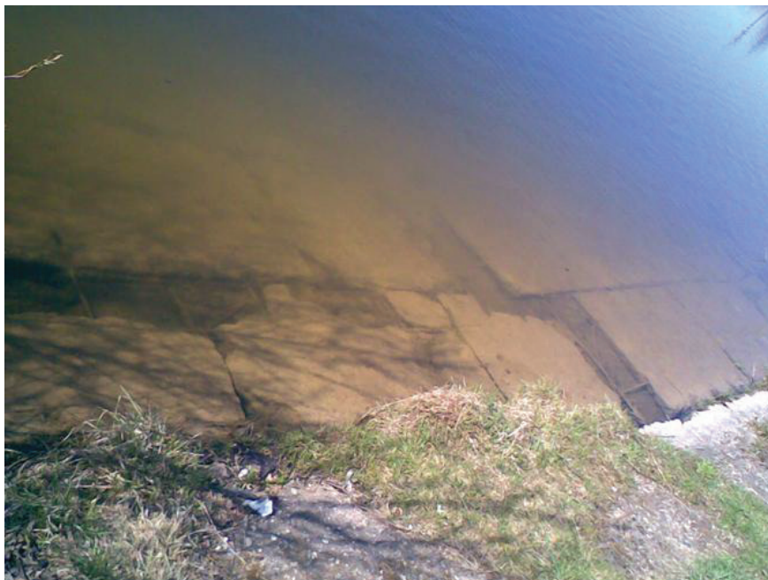
Figure 1: Destroyed slabs for ponds slope protection in zone B.
