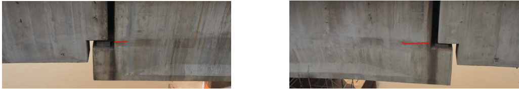
a) Cracks at Dechatiwong Bridge No.2 b) Cracks at Dechatiwong Bridge No.3 Figure 1: Ledge girders and horizontal crack at reentrant corner in Dechatiwong Bridge.
