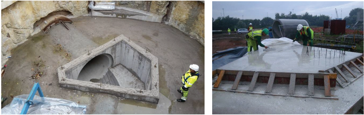
Figure 3: Inspection pit (left) and roof plate made of self-healing concrete with MUC+ (right)
