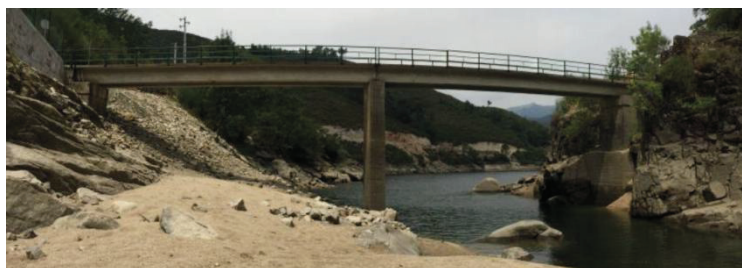
Figure 1: Overall view of Saltadouro Bridge (left side: North abutment; right side: South abutment).
