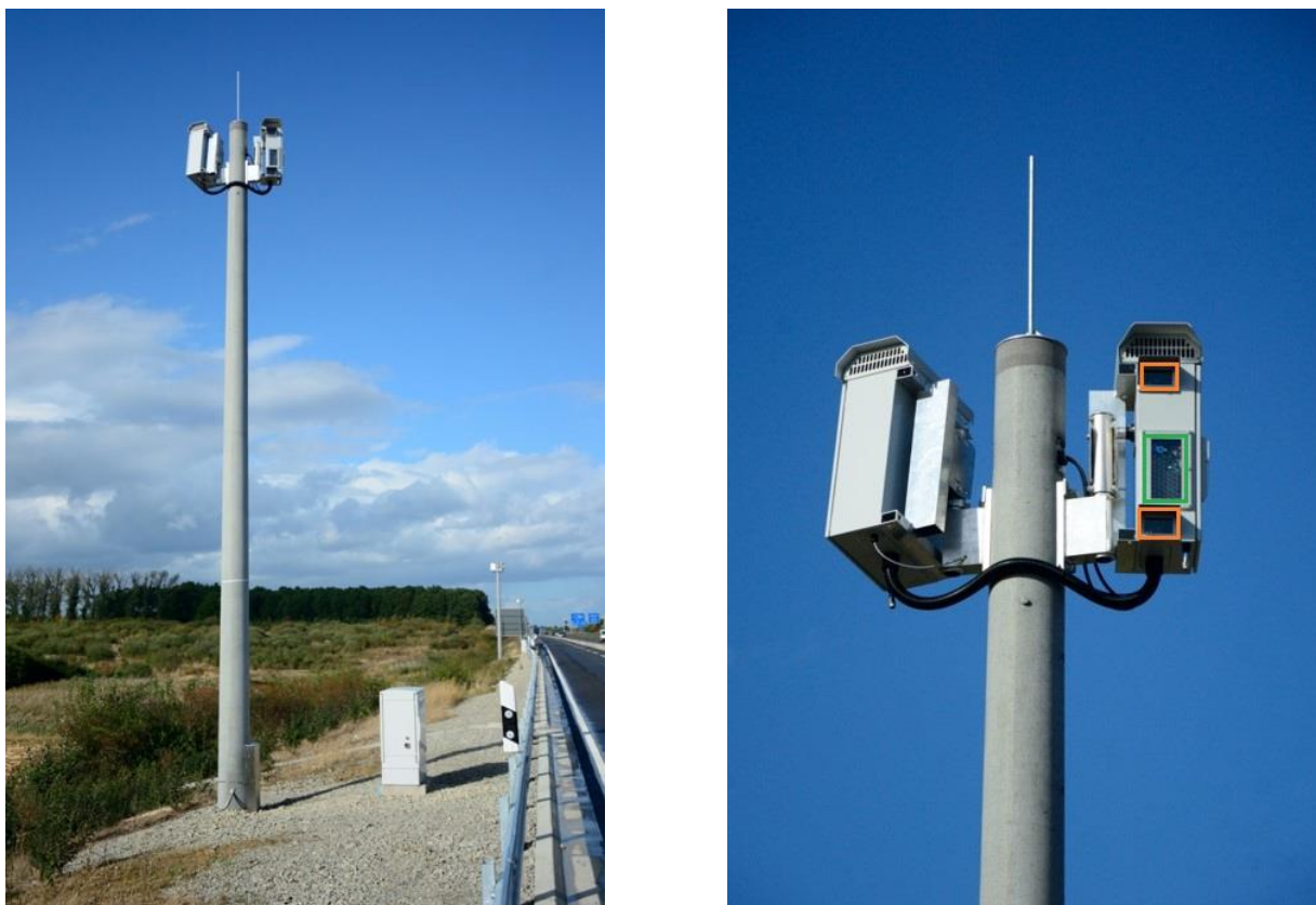
Figure 5: Multi-sensor system mounted on pole next to the A39 highway, cameras and infrared lighting highlighted
