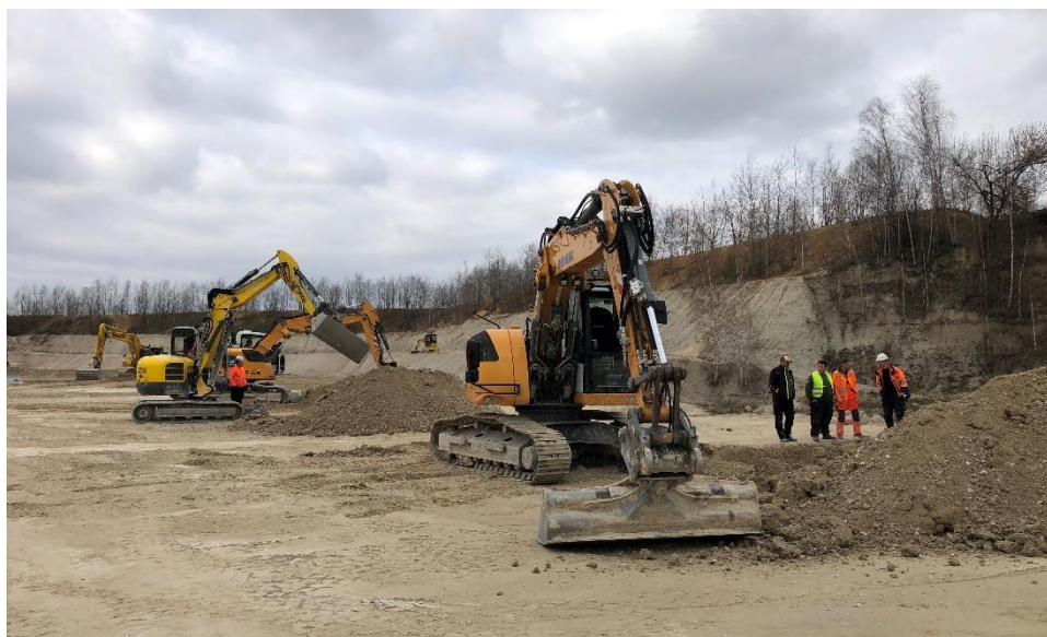
Figure 26: Picture from the visit to Glauchau in March 2024, where the first UC3 co-design workshops with experienced excavator operators and apprentices took place
