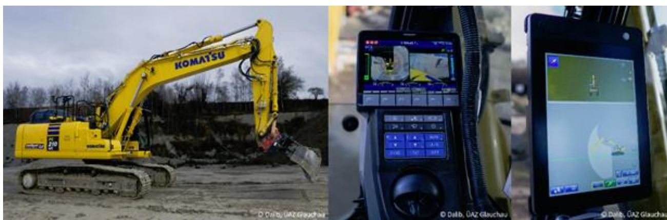
Figure 26 An excavator with a 3D-machine control system and a bird-view camera setup in order to monitor the danger areas close to the machine (© ÜAZ Glauchau, Bau Bildung Sachsen e. V.)
