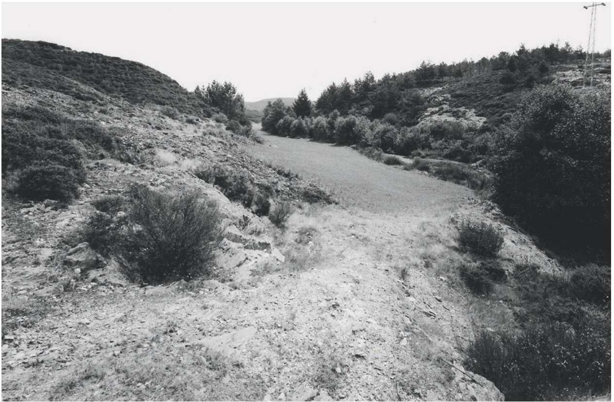
Fig. 5.0-8: Territorium metallorum Tresminas / Jales, from the west: Outeiro earth fill dam. Both preserved wings are recognizable (photo: J. Wahl).
