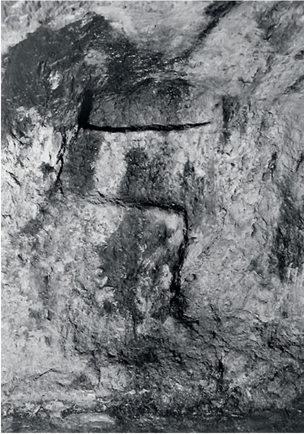
Fig. 3.3.1-20: Territorium metallorum Tresminas/Jales, Tresminas, Galeria dos Morcegos: working face, the cutting of the rock went from the top down, as the various steps of the cuts show (photo: J. Wahl).
