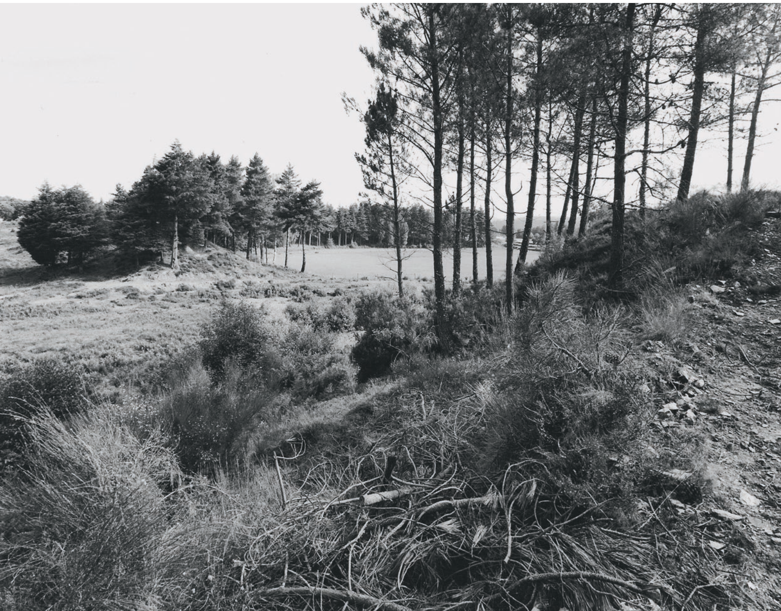
5.0-10: Territorium metallorum Tresminas / Jales, from the westsouthwest: Outeiro earth fill dam, with rock base and heaped earth (photo: J. Wahl).
