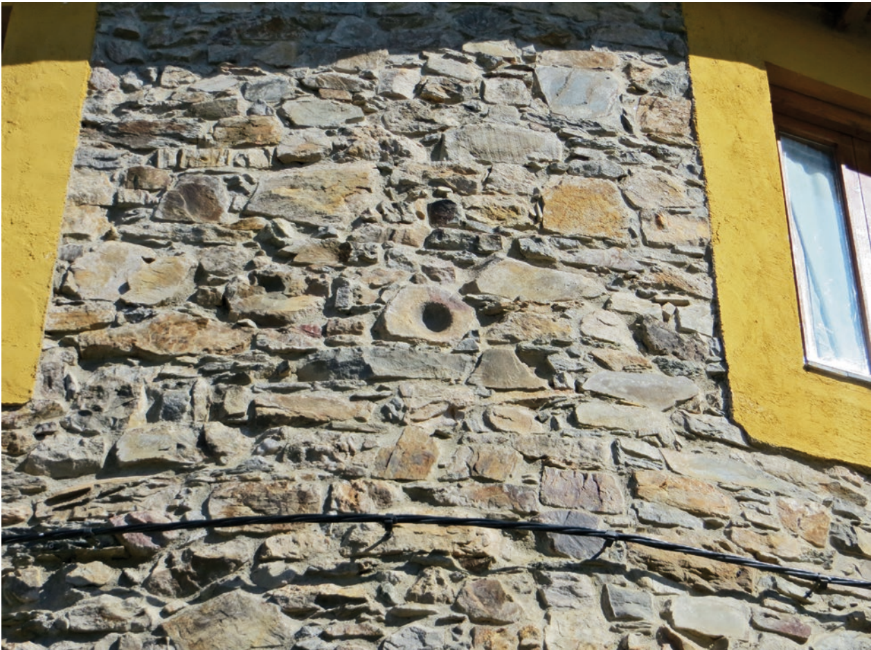
Fig. 4.0-21: Pozos (Prov. León / E): heavily used stamp mill base for a single stamp, reused in the construction of a house (photo: R. Wahl-Clerici).
