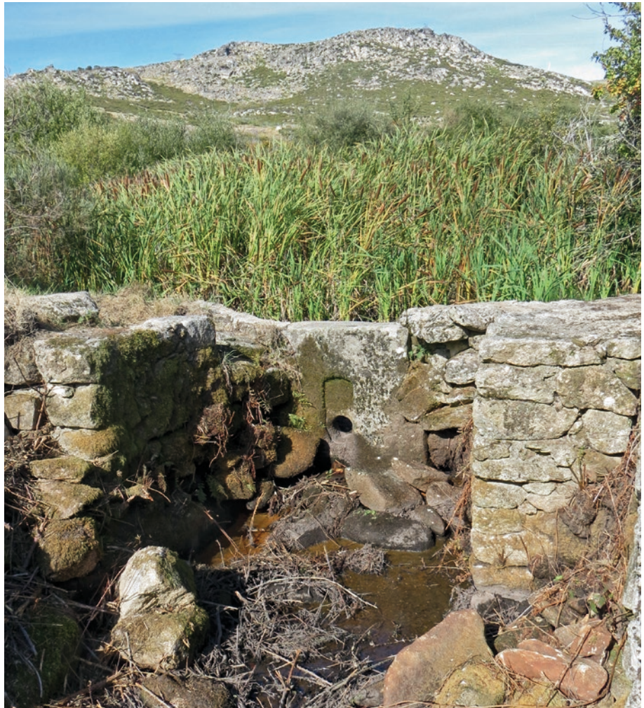
Fig. 5.0-19: Territorium metallorum Tresminas / Jales: rockfill dam on the upper reaches of the Ribeiro da Peliteira with the bottom outlet with the regulating stone, as seen from the valley (photo: R. Wahl-Clerici).
