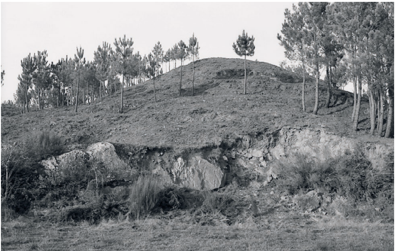
5.0-9: Territorium metallorum Tresminas / Jales from the west: Outeiro earth fill dam. In the foreground, the rock used as base is visible (photo: R. Wahl-Clerici).
