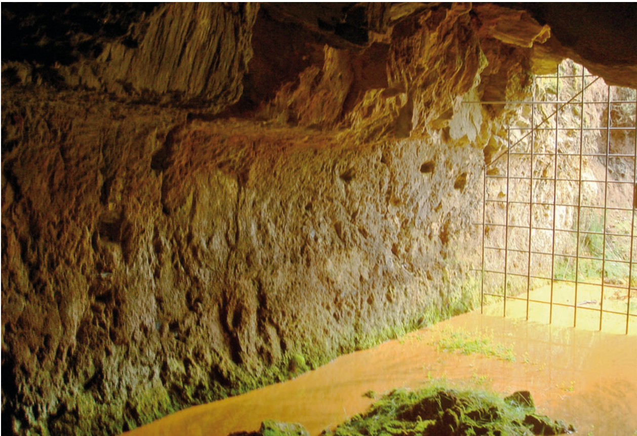
Fig. 3.3.1-6: Territorium metallorum Tresminas / Jales, Tresminas, Galeria dos Morcegos: entrance area, with niches for lamps visible in the vertical western workforce, which were necessary during the driving of the pilot drift into the rock. The roof is only in part in its original state, as it collapsed several times (photo: R. Wahl-Clerici).
