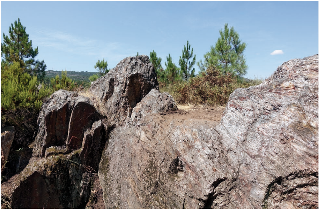
Fig. 3.0-31a: Territorium metallorum Tresminas / Jales, Gralheira; from the southeast: a completely collapsed former open pit mine with the remains of an entrance in the northern working face (photo: R. Wahl-Clerici).
