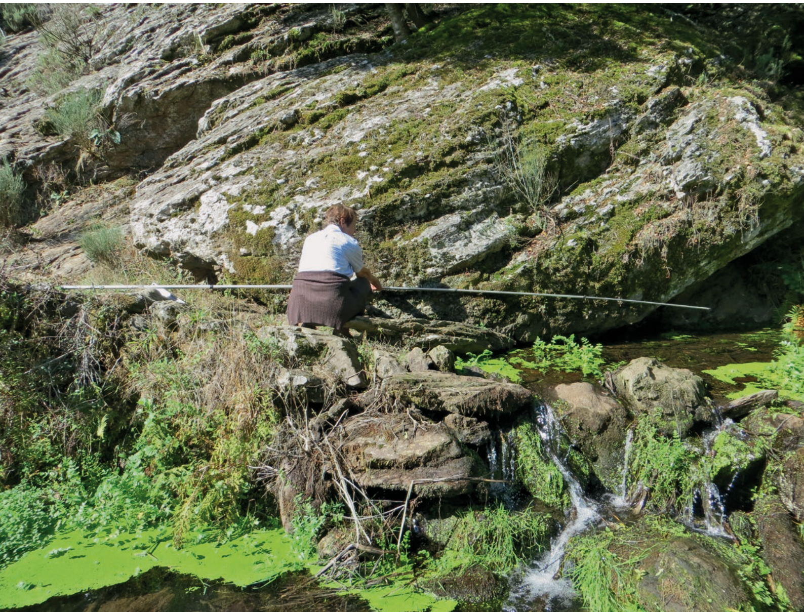
Fig. 5.0-21: Territorium metallorum Tresminas / Jales: Sevivas weir, the measuring stick indicates the level of the C4-aquaeduct (photo: R. Wahl-Clerici).
