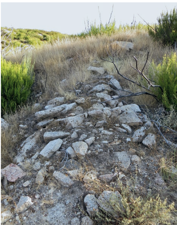
Fig. 5.0-12: Territorium metallorum Tresminas / Jales: detail on the southern side of the rockfill dam on the upper reaches of the Ribeiro da Peliteira (photo: R. Wahl-Clerici).
