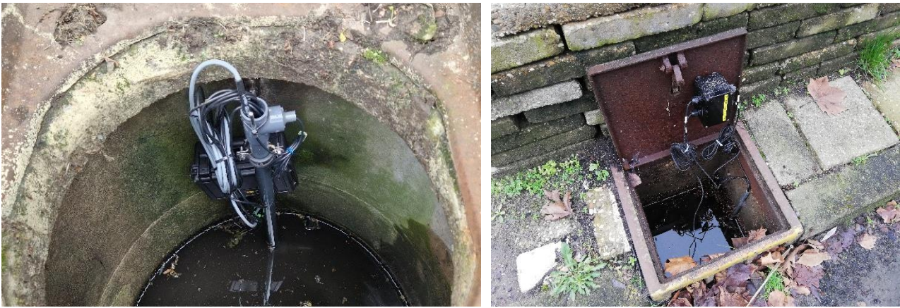
Figure 1. Photos of the MONTSE devices installed in gully pots in Dübendorf (left) and Delft (right).
