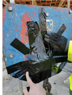
Figure 4 sensors mounted on a crane hook
