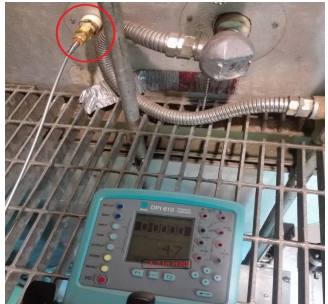
Figure 1 – 11NMC Inlet Casing Differential Pressure port for performance analysis
