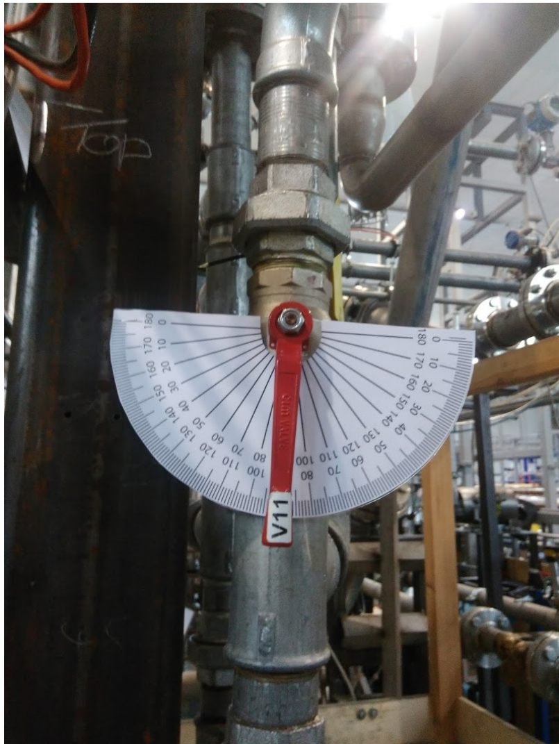
Figure 8. Manual valve V11 used for simulating air blockage
