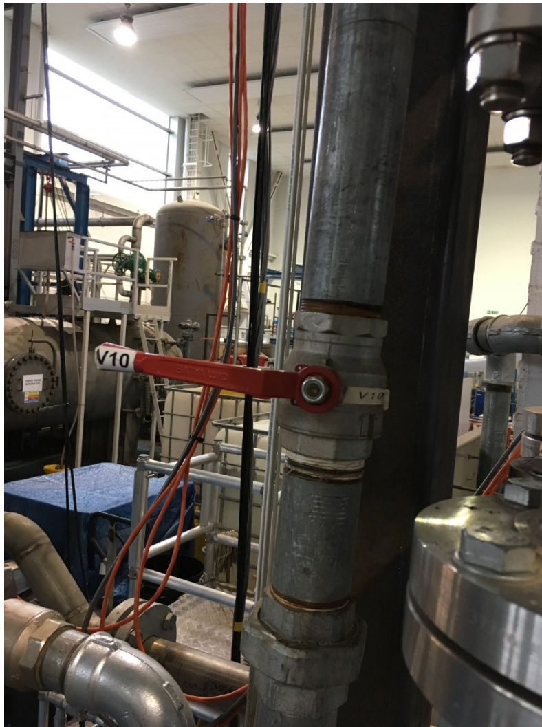
Figure 7. Manual valve V10 used for simulating air leakage
