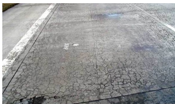
Fig. 1 Damage of top layer of the concrete road with RCA due to ASR
