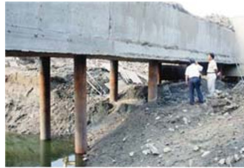
Fig. 1 Example of embankment failure by piping
