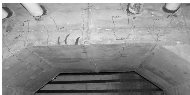
Fig. 3 (a) Actual view of anchor beam cracks
