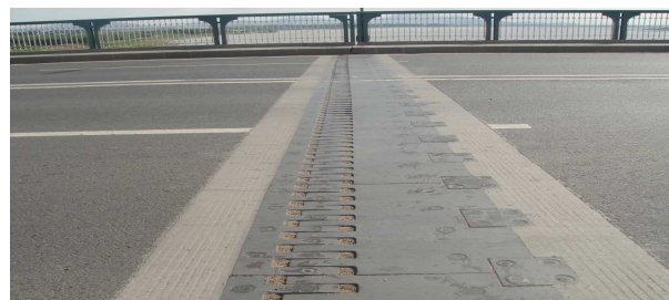
Fig. 4 (a) Joint fill with dust
