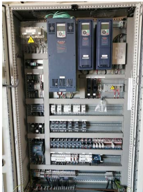
Figure 17. RO plant main panel, with the VFDs of the HPP, booster pump and CIP pump.
