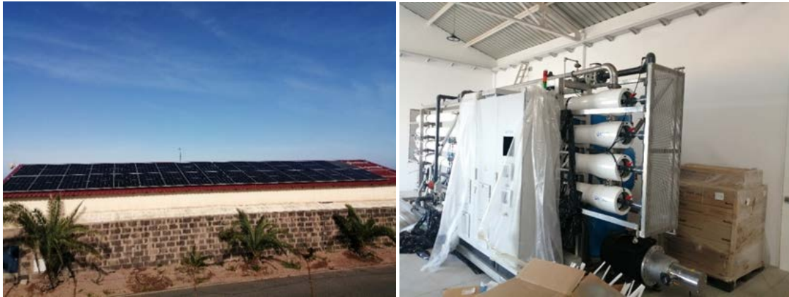
Figures 15 and 16. PV field on the roof of the building and SWRO desalination plant.
