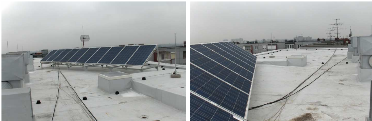
Photovoltaic panels on the top of the retrofitted multi-storey house at Mierová 1436
