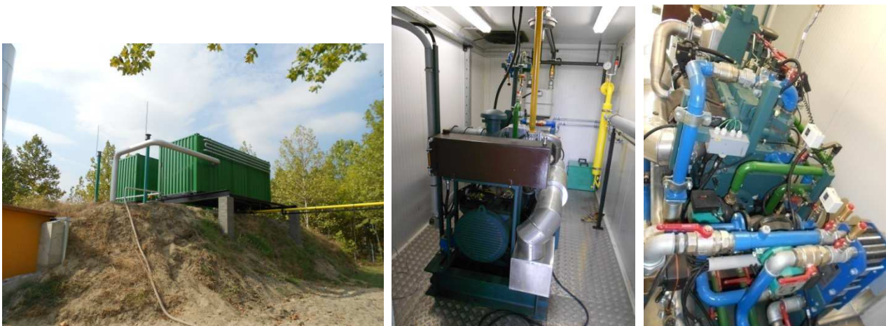
One of the two waste-gas (methane) fuelled CHP engines at Mórhalom
