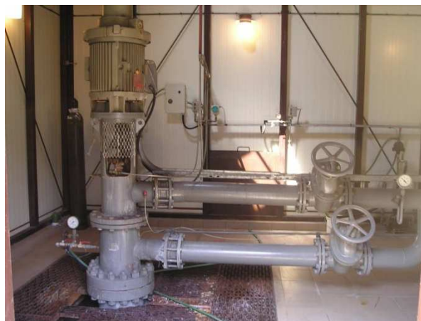
Well-head of the Galanta geothermal abstraction well
