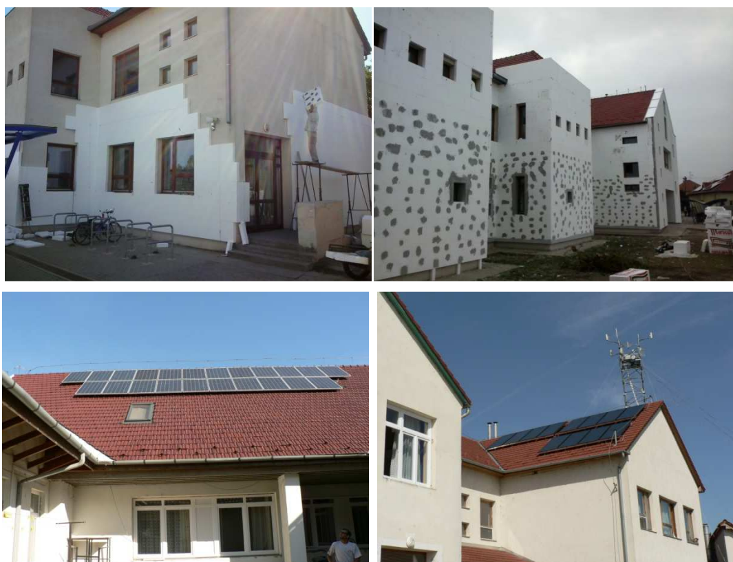
Step-by-step facade insulation and the installed solar-thermal collectors at both target buildings
