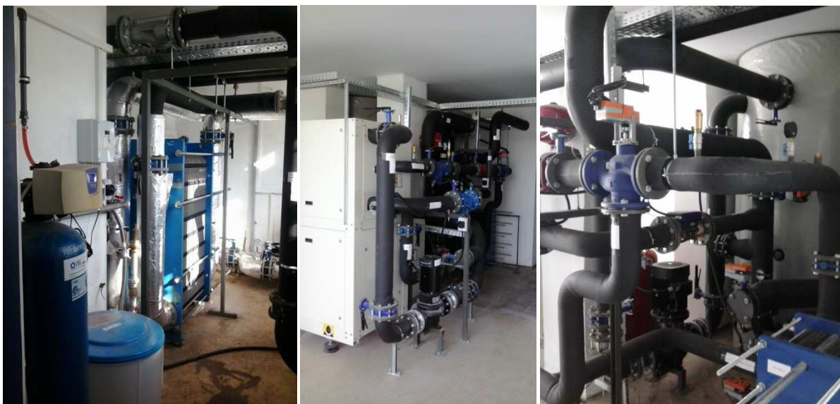
The engineering components of the high power heat pump station at Mórahalom
