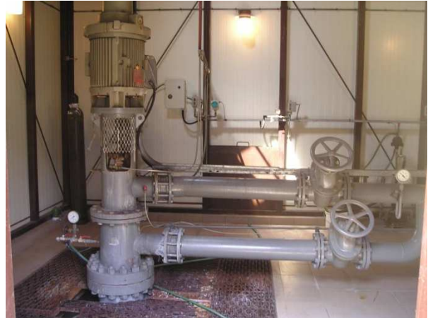
Well-head of the Galanta geothermal abstraction well
