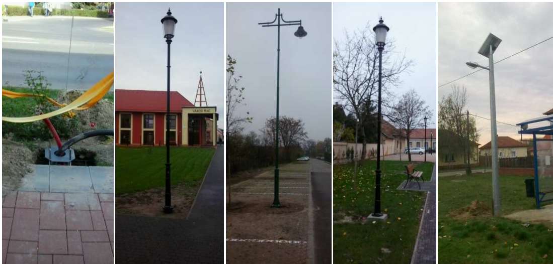
Different types of public lamp post accommodating the LED lighting fixtures at Mórahalom
