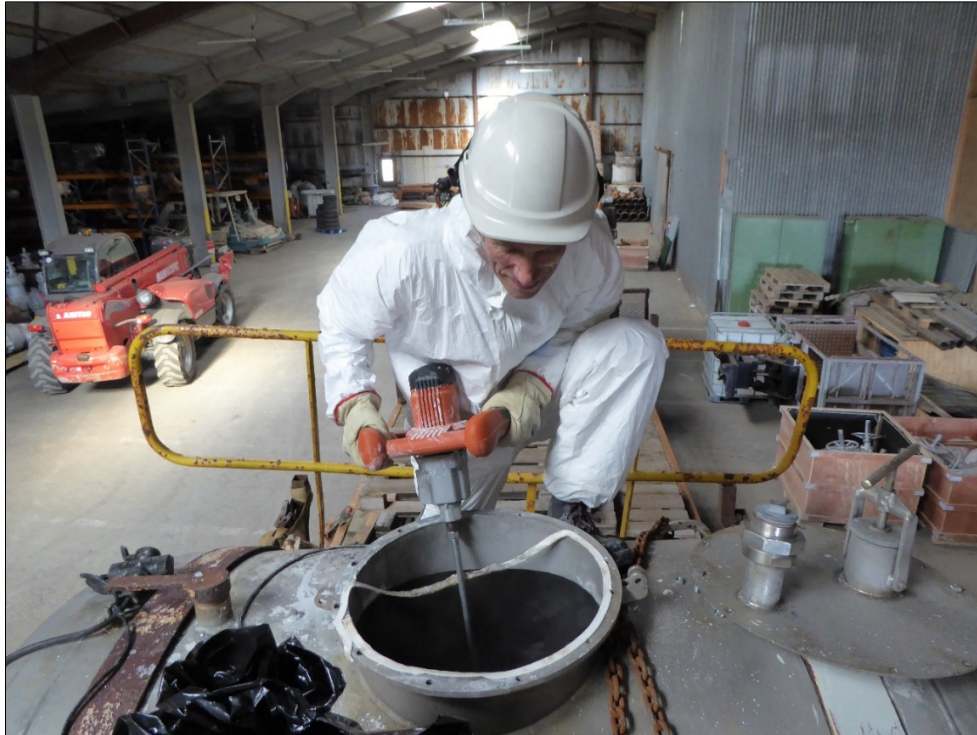
Figure 4. Dissolving the tracer in the tank by stirring with the help of the electric stirrer.
