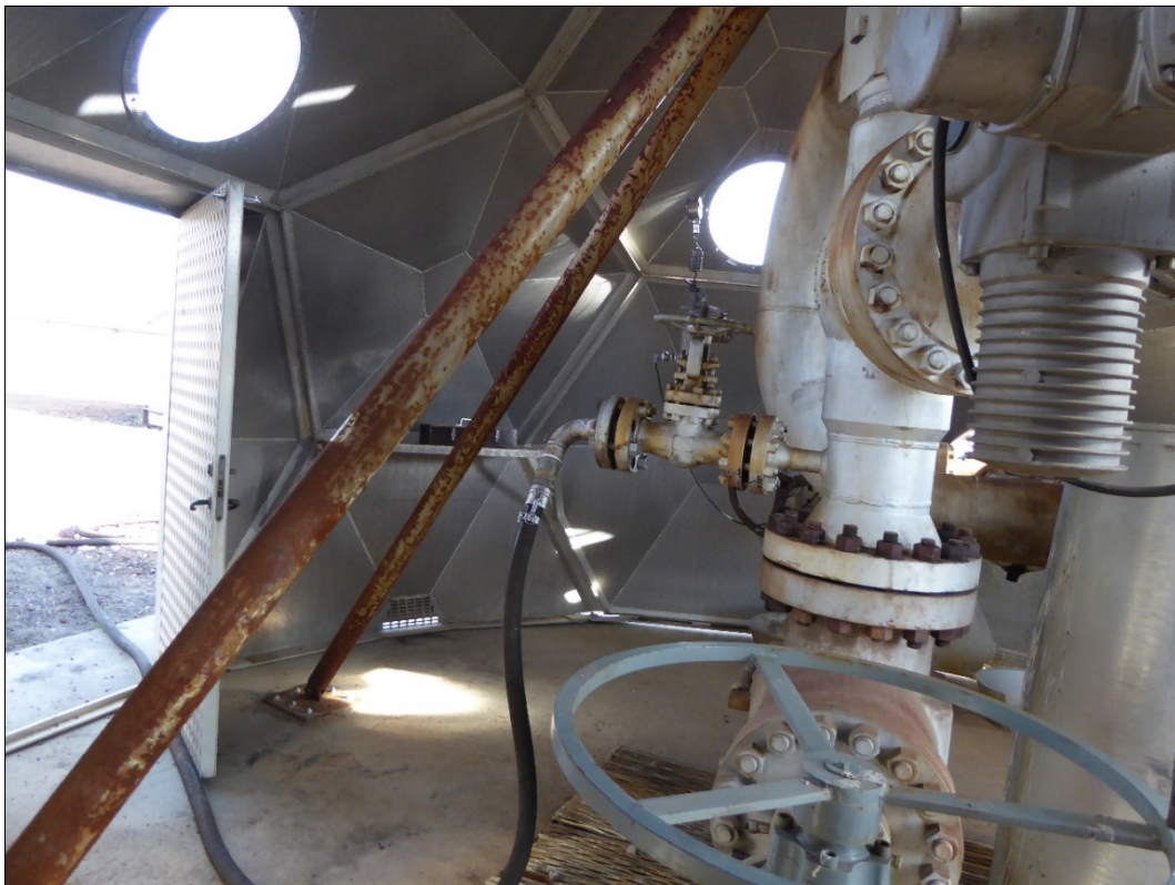
Figure 7. Injection of the tracer through the black pipe into well KJ-39 using the pump.
