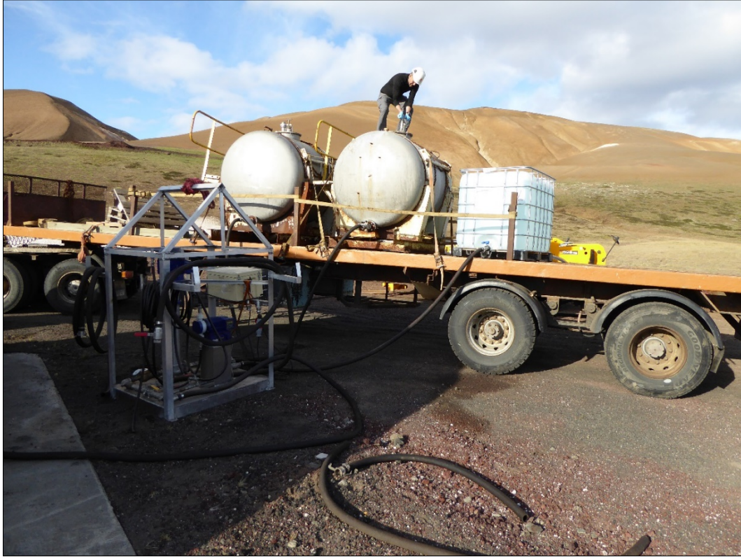
Figure 6. The pump and the trailer with the tanks and clean water in front of well KJ-39.
