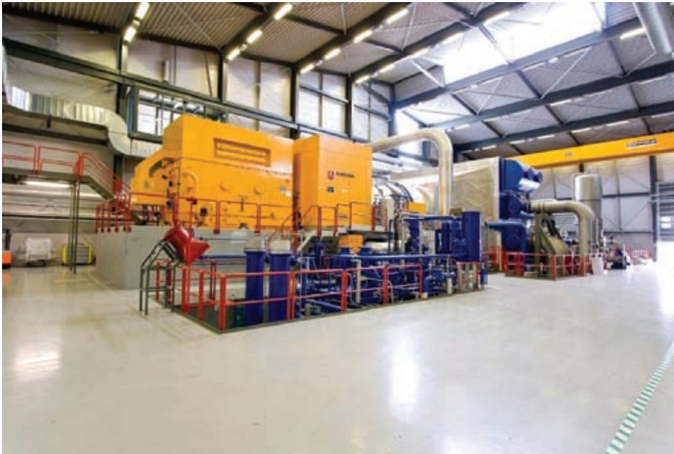
Figure 3. Machine hall of Hellisheiði Power Plant
